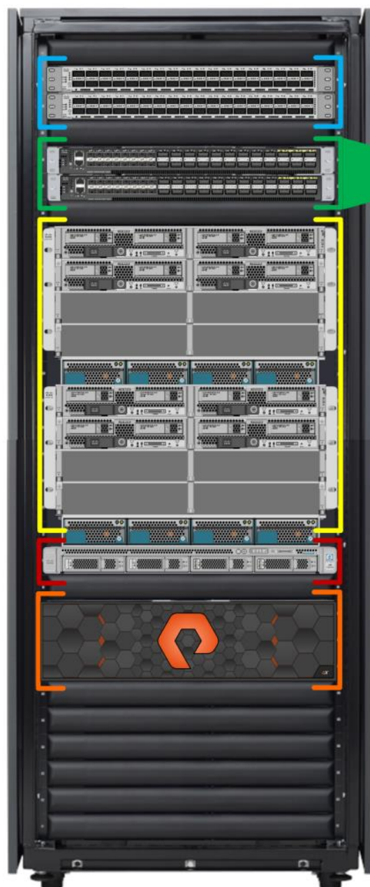
Figure 5 Configuration Overview of the Cisco UCS Infrastructure
