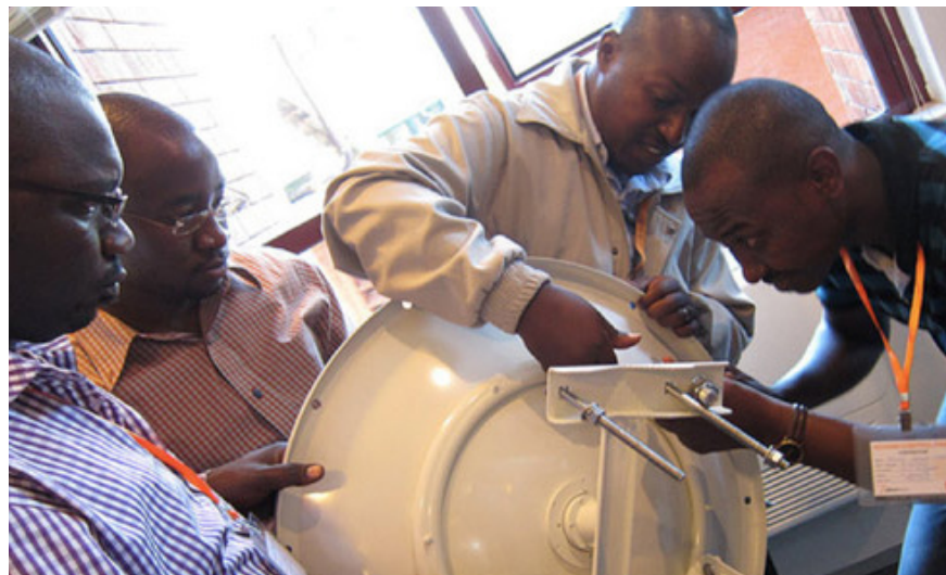
[photo left] Trainees from Orange Kenya, Inveneo ICIP, Setright, and Dadaab-based IT staffs assemble an Ubiquiti Rocket Dish.
