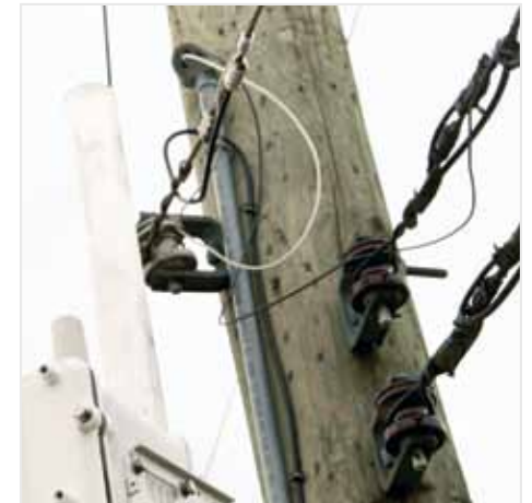
Improved the quality of power supply
