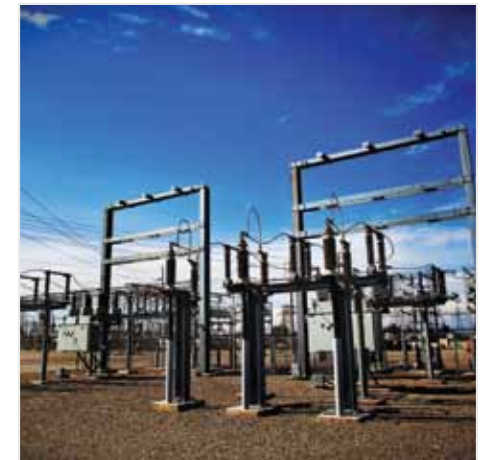
Improved the quality of power supply
