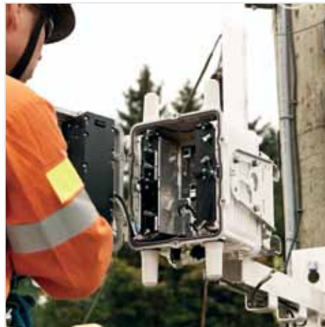
Shortened fault identification, fault isolation and power restoration time
