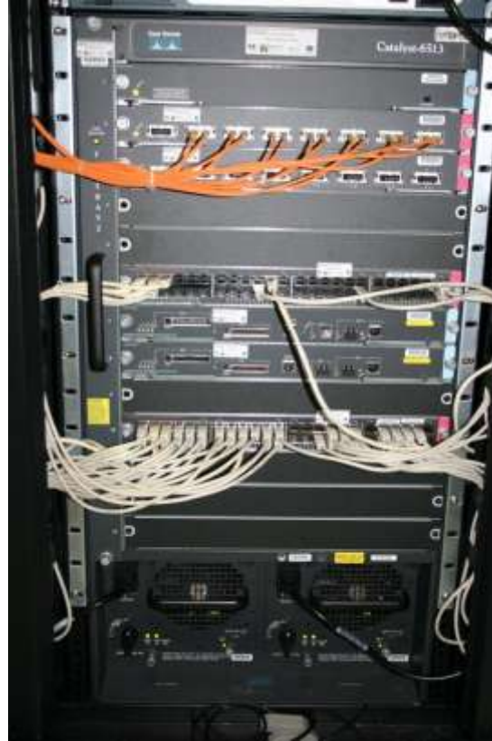
Switch Core Cisco Catalyst 6513
