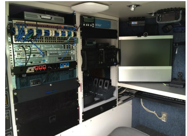
Figure 2: The engineering section of the Cisco MCV brings together complementary technologies and solutions to provide situational awareness for the command staff.
